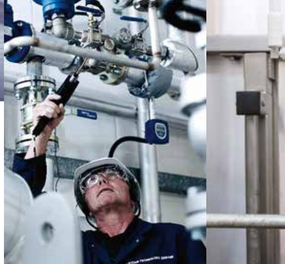
Manuele controle condenspotten. (Foto Spirax Sarco)
